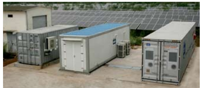
Fig. 3 : A view of the containerized 1 MWh BESS
